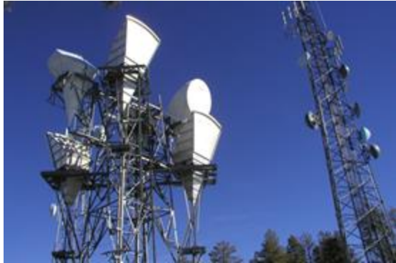
Telecommunications Mobile Backhaul
